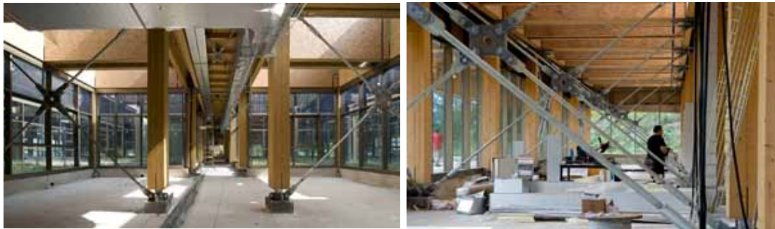
Figure 4: Views into the courtyards and site while under construction: (Moreno Maggi Photographer, MCA, 2017)
